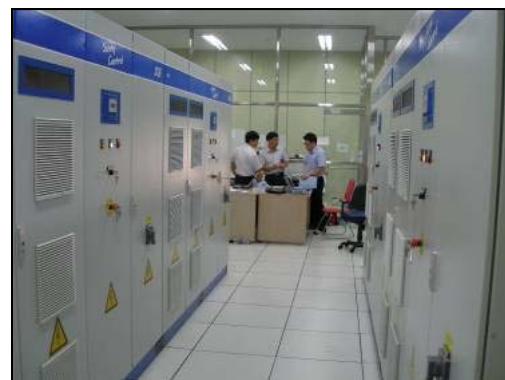
Control room with inverters and Sunny Team
