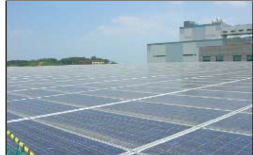
Solar array with thermal power station in background.
