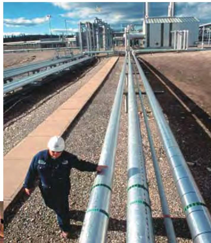
As part of regular maintenance, an employee at the BP gas processing plant in Ricinus, Alberta inspects pipeline.
