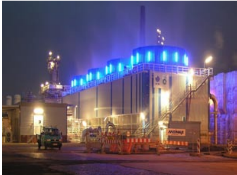
In 2005 the operating permit for the new cooling plant in Horst was issued
