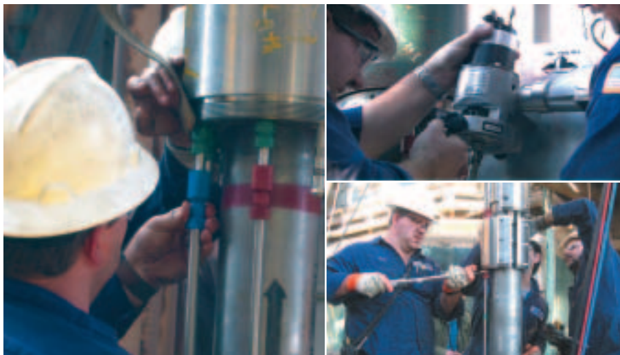
Installing and connecting hydraulic and electrical control lines for a well has always been a tough and potentially hazardous procedure. The Thunder Horse completions team has improved this operation by developing a new suite of blade-free cutting, bending and connection-making tools
