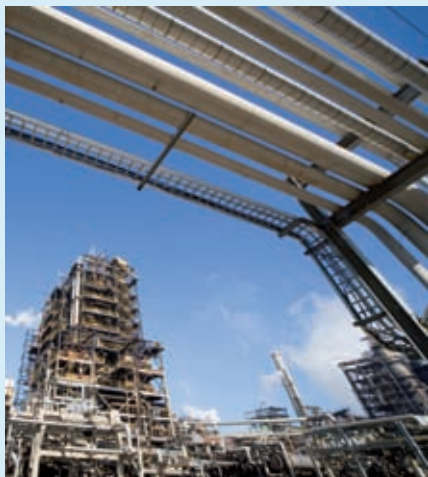
In the planned upgrade of BP's Whiting refinery (above), vacuum residue from heavier crude oil feedstock will be treated in a 'delayed coking' process (right) to produce additional transportation fuels, and petroleum coke
