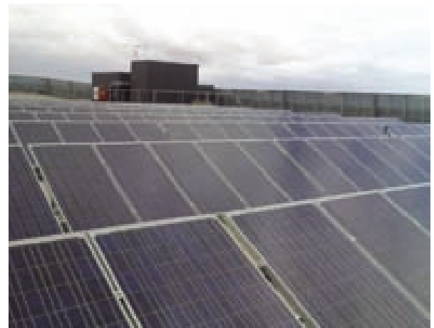
The solar system is located on the top floor of the Bus Station's car park and comprises of 320 solar panels.
