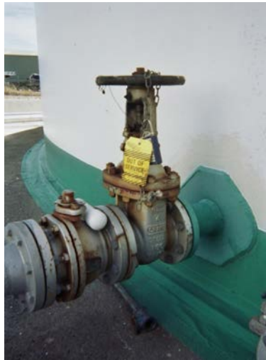
Figure 1: Single Valve Isolation with Lock and Tag
