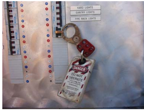
Figure 2: Electrical Circuit Breaker with Multiple Lock hasp, Single Lock and Tag
