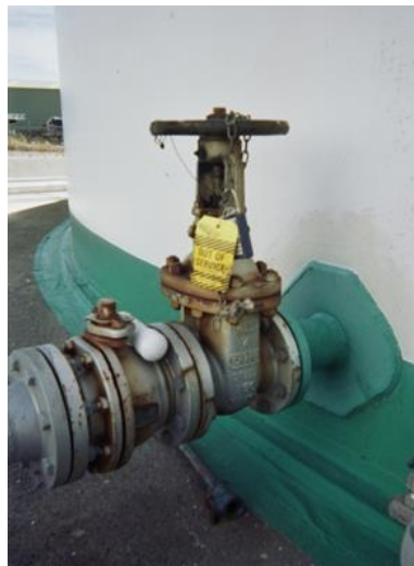
Figure 2: Single Valve Isolation with Lock and Tag
