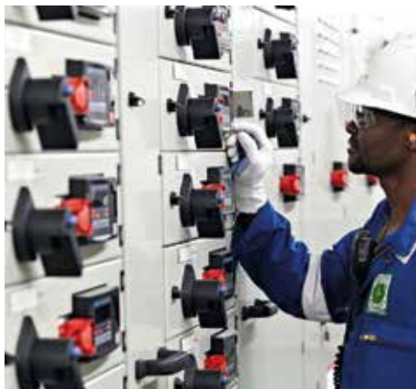
▲ A technician in the electrical room onboard the FPSO.
