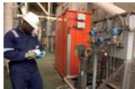
Greater Plutonio FPSO plant area
