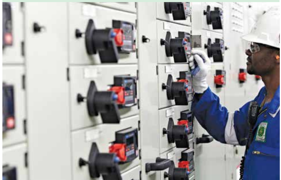
▲ An Electrical Technician at the FPSO Greater Plutonio electrical room.
