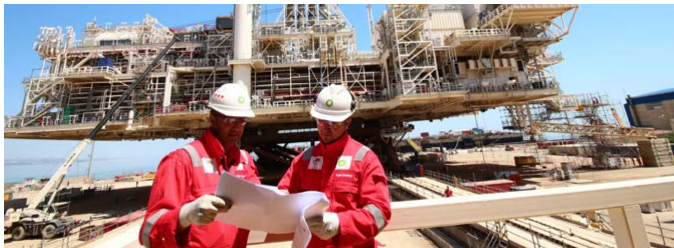
Caption: Workers discuss work plans at the Shah Deniz 2 platform quarters and utilities topsides unit which was installed offshore in July 2017.
