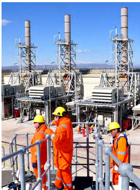
BTC pump station 1 in Georgia.
