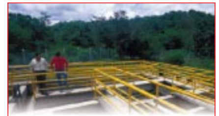
The provision of a complete water treatment and distribution system in Colombia delivered greatly improved health standards:
