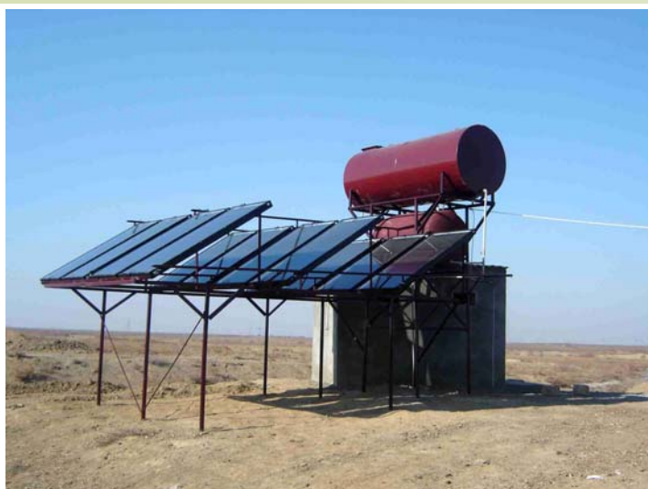
Water tank for hot water
