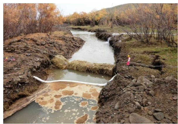
After: Straw bales installed to filter out turbid water before mixing with the river flow
