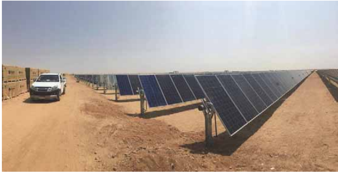
Figure 3.10: PV modules installed on a single axis tracking system
