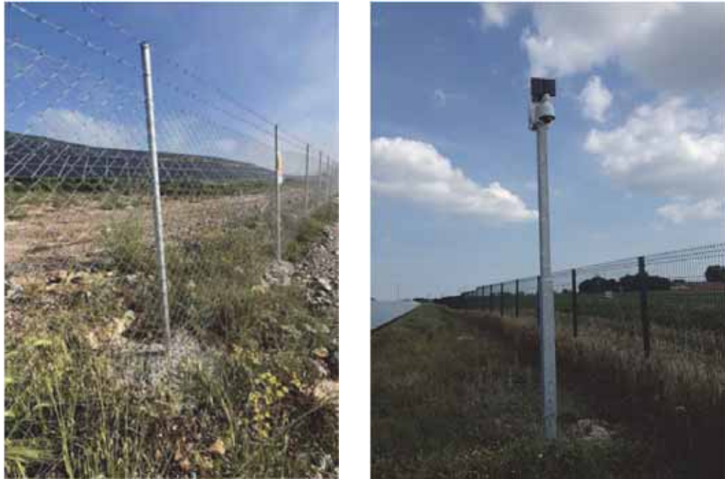
Figure 3.15: Example of typical security fencing and CCTV
