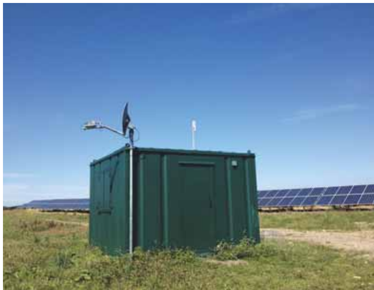
Figure 3.14: Example of a communications building
