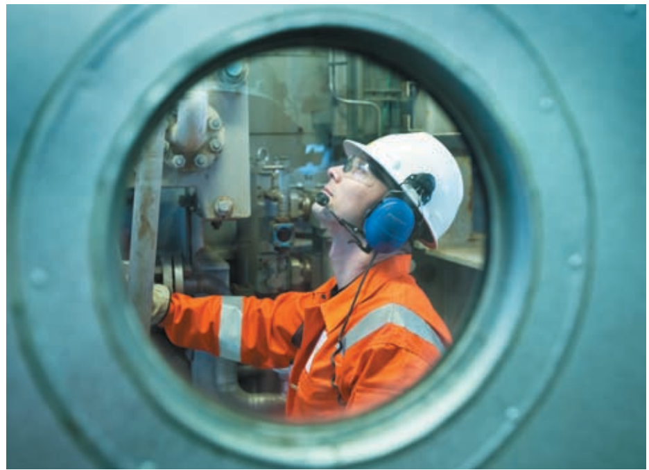
Power turbine inspection on East Azeri platform
