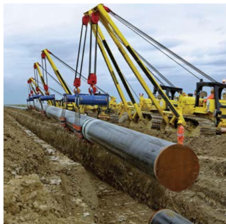
Left: Pipe lowering activity in Hajigabul district as part of the South Caucasus Pipeline expansion project. Right: Construction of Shah Deniz Stage 2 platform topsides is well underway.
