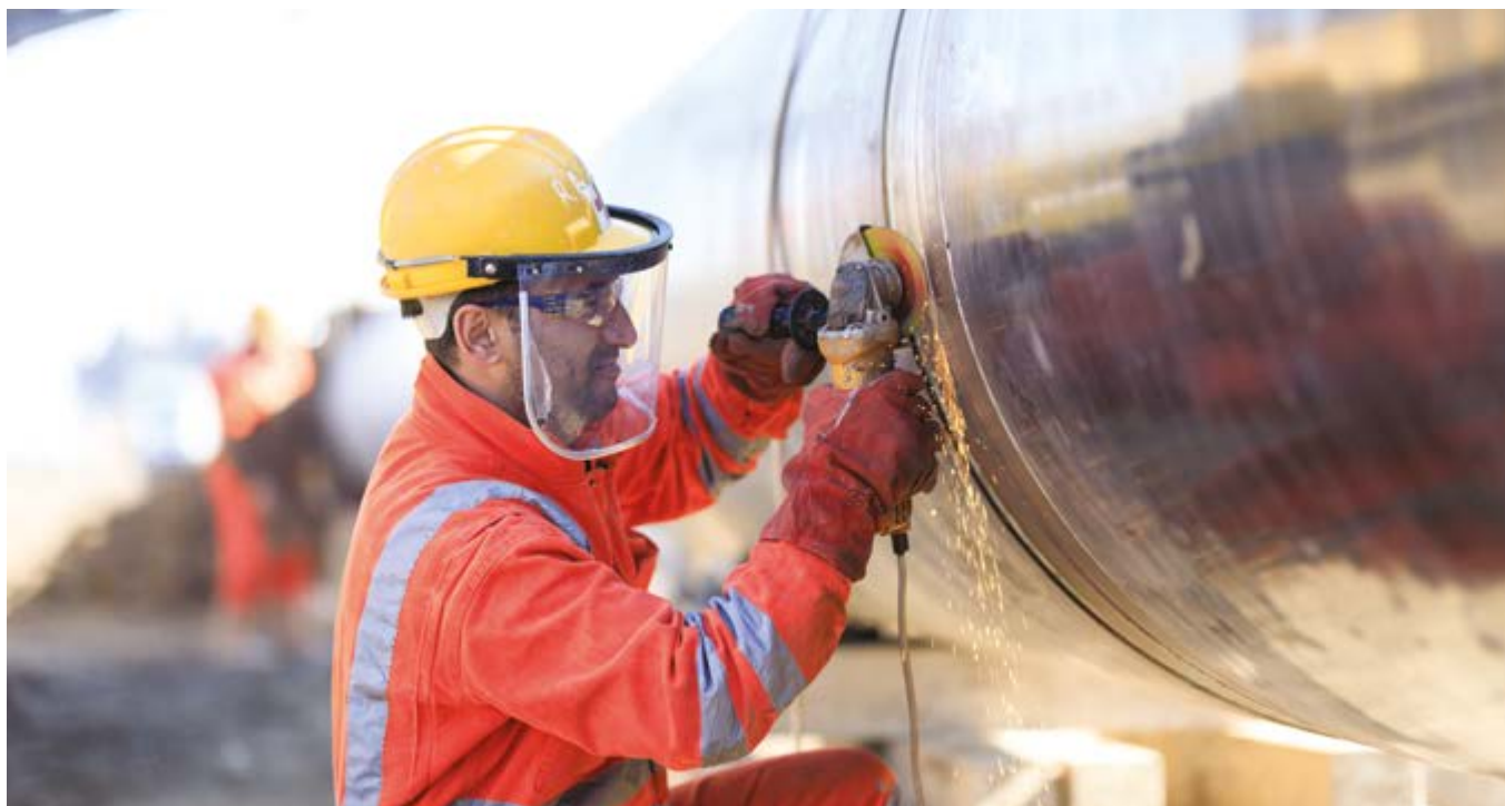
Worker grinds a pipe section for the South Caucasus Pipeline construction works.
