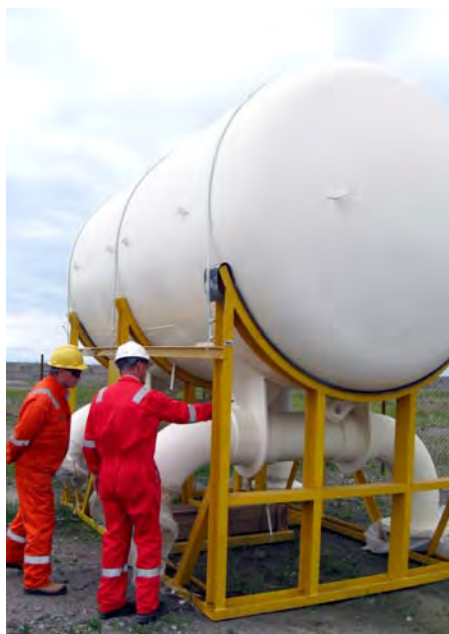
Mid water buoyancy tank, Supsa Terminal
