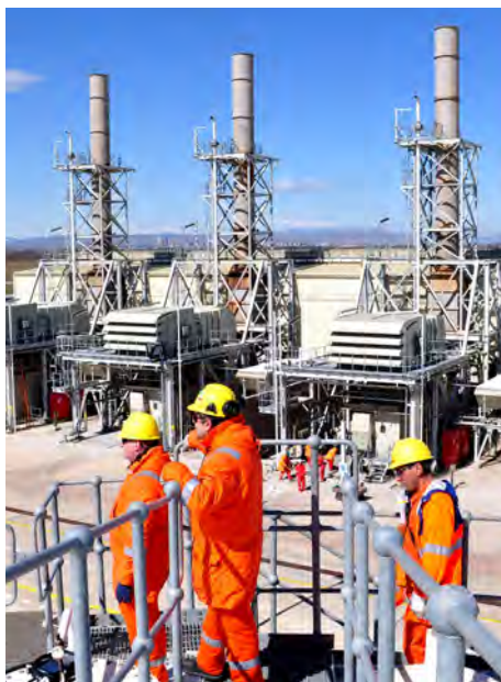
BTC pump station 1 in Georgia.
